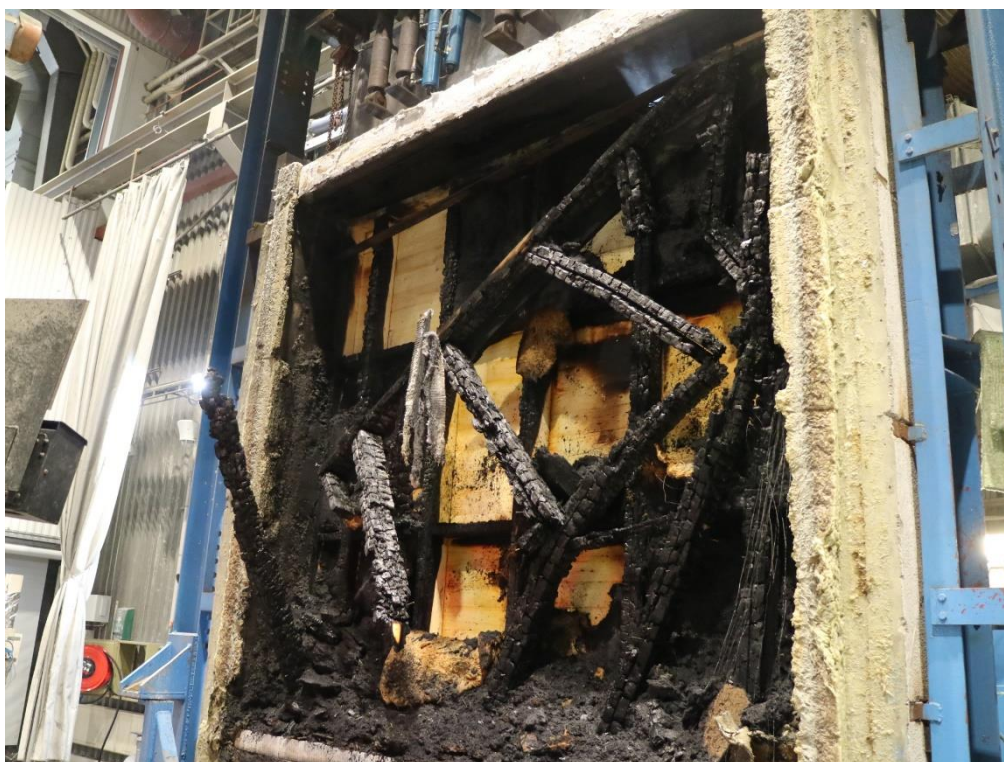
Fire exposed side after the test.
